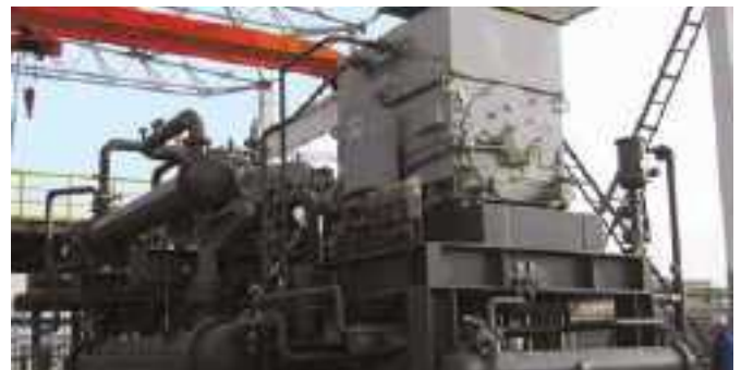
A centrifugal gas compressor for CO compression
